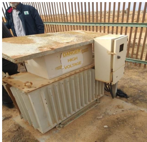
Figure 6: Transformer rectifier at Tobruk station
